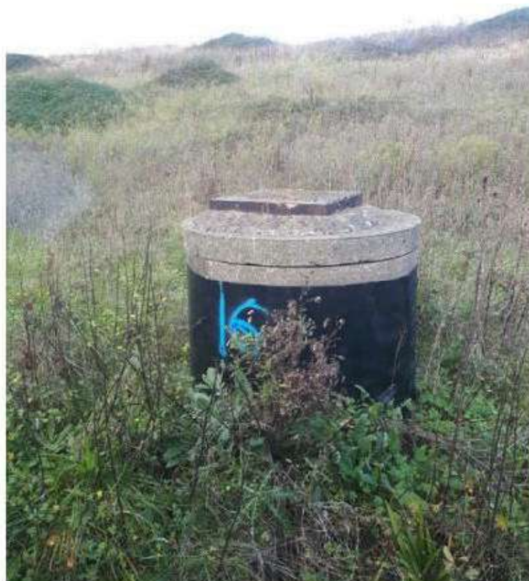
Figure 5: Example of gas infrastructure at former Lamby Way Landfill site.
